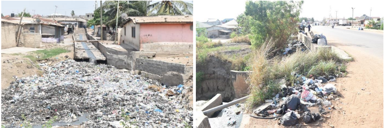
Picture 5.3 Accumulation of garbage in the Drains at Ashaiman
